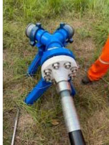
CONEXION FRACK TANK
